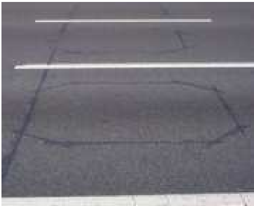
Figure 1: inductive loop sensors
